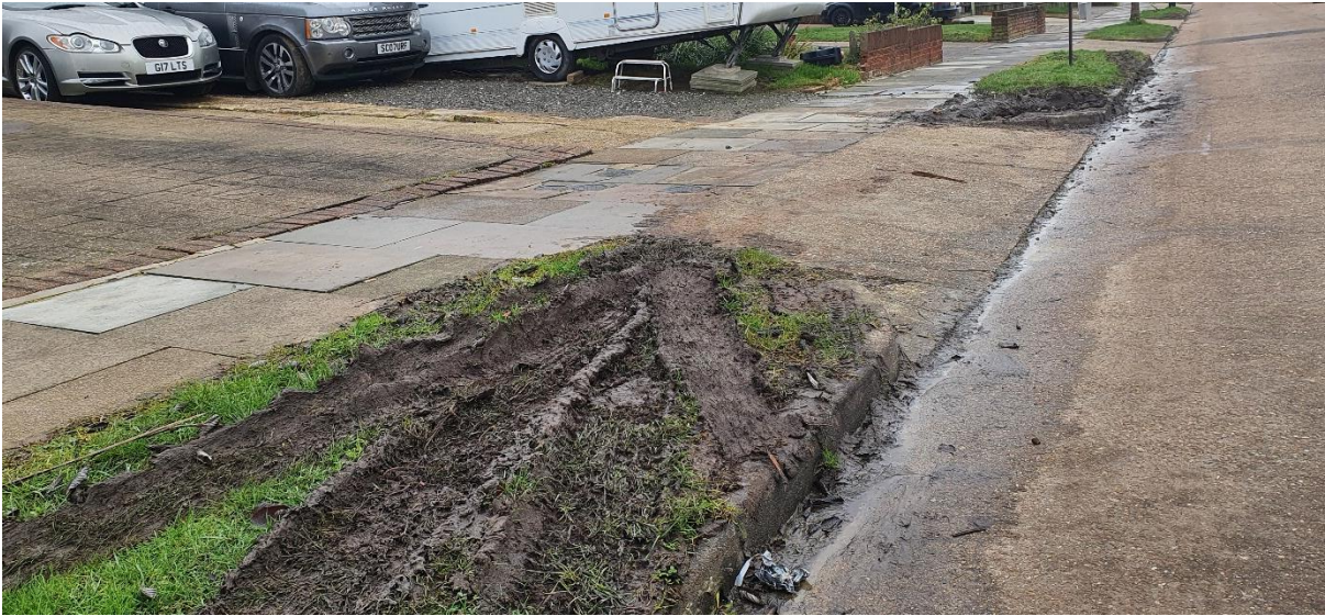
Figure 14 – example of damage to grass verges
